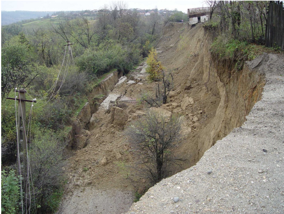
Figure 3. The landslide occurrence affecting surface infrastructure, power lines and roads, example of the Lăpușata commune (6 November 2004), Vâlcea County.
