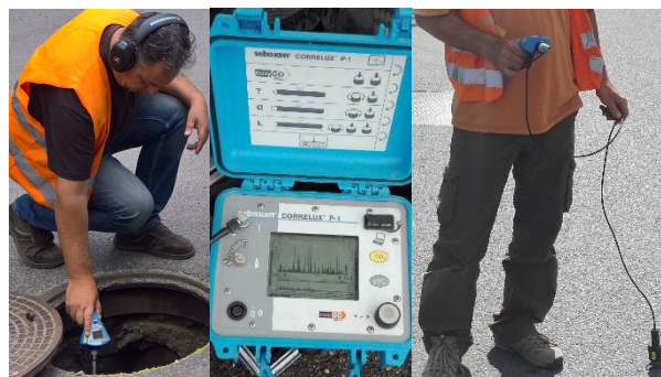
Figure 13. Leak locator (left and right) and Digital correlator for leak location on pipe (middle).
