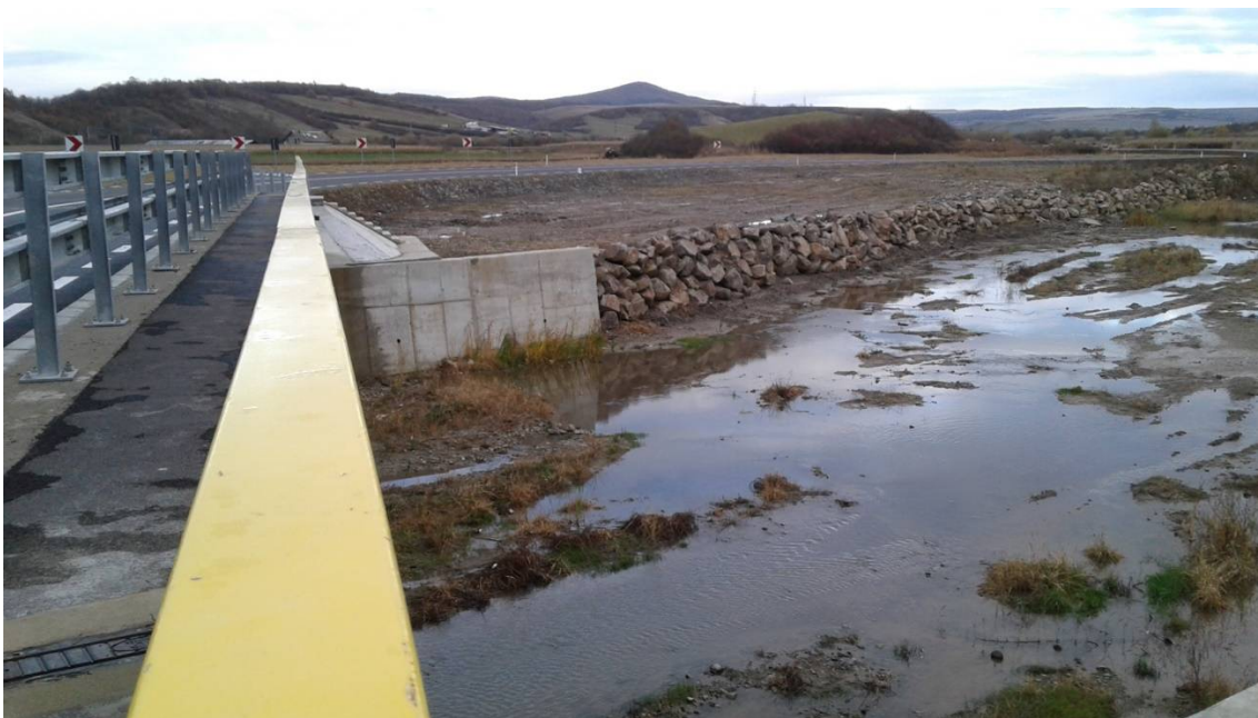
Figure 7. The right bank of Şieu river after the bridge construction (photo by Claudiu Gavriiloaie).
