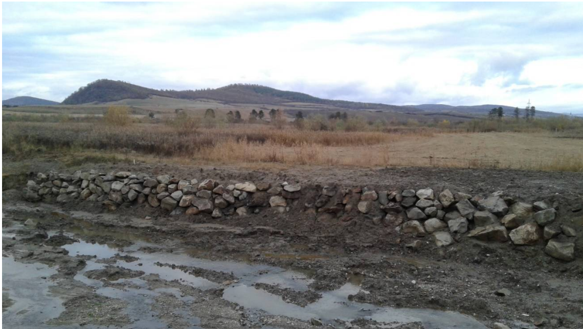
Figure 8. The left bank of Șieu river after the bridge construction (photo by Claudiu Gavriiloaie).
